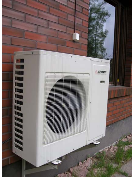
Air Source Heat Pump (ASHP)
