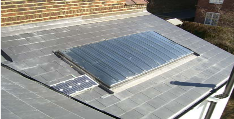
Solar thermal (hot water) panel Picture Credit: www.ecorefurbishment.co.uk
