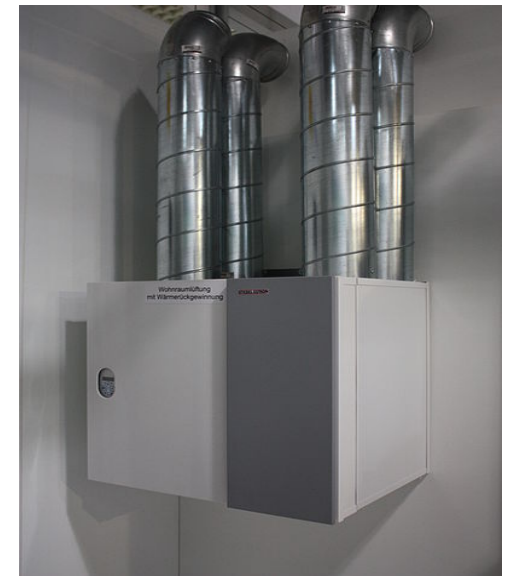
Mechanical Extract Ventilation (MEV) Unit
