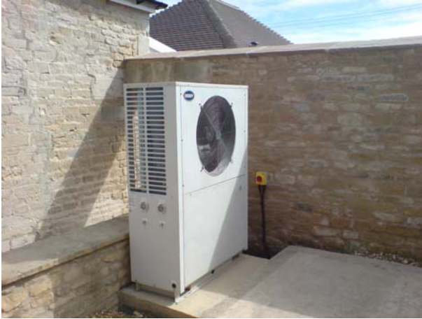
Air Source Heat Pump (ASHP) Picture Credit: Radiant Heating Solutions Ltd
