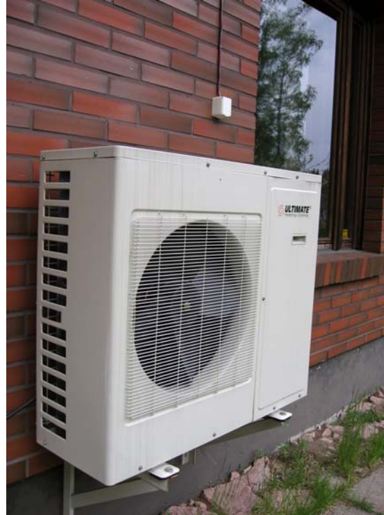
Air Source Heat Pump (ASHP)
