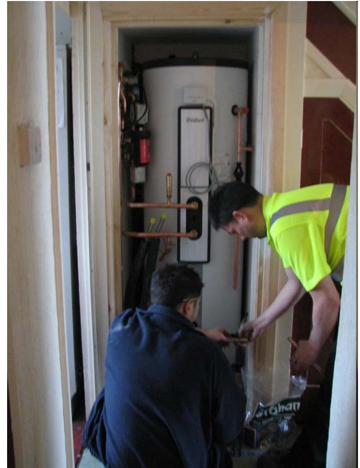
Twin coil water cylinder in solar thermal system Picture credit: Bere:architects
