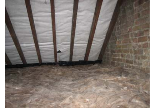
Insulation installed between and over joists in loft. Picture credit: ECD Architects
