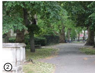
Deteriorating path edges
