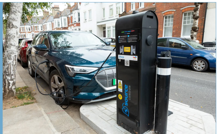
Figure 3: Example of an electric vehicle charging point.
