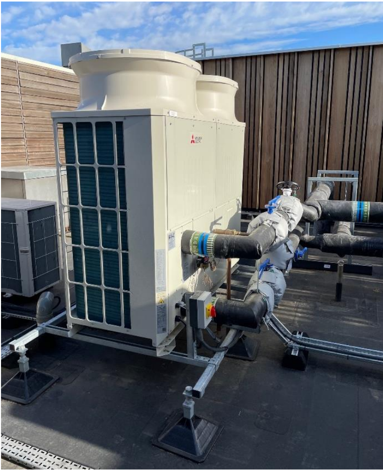
Figure 24: An air source heat pump installed at Talacre Community Sports Centre. This has replaced a gas boiler and will therefore reduce climate impacts whilst also helping to improve local air quality and protect community health and wellbeing.
