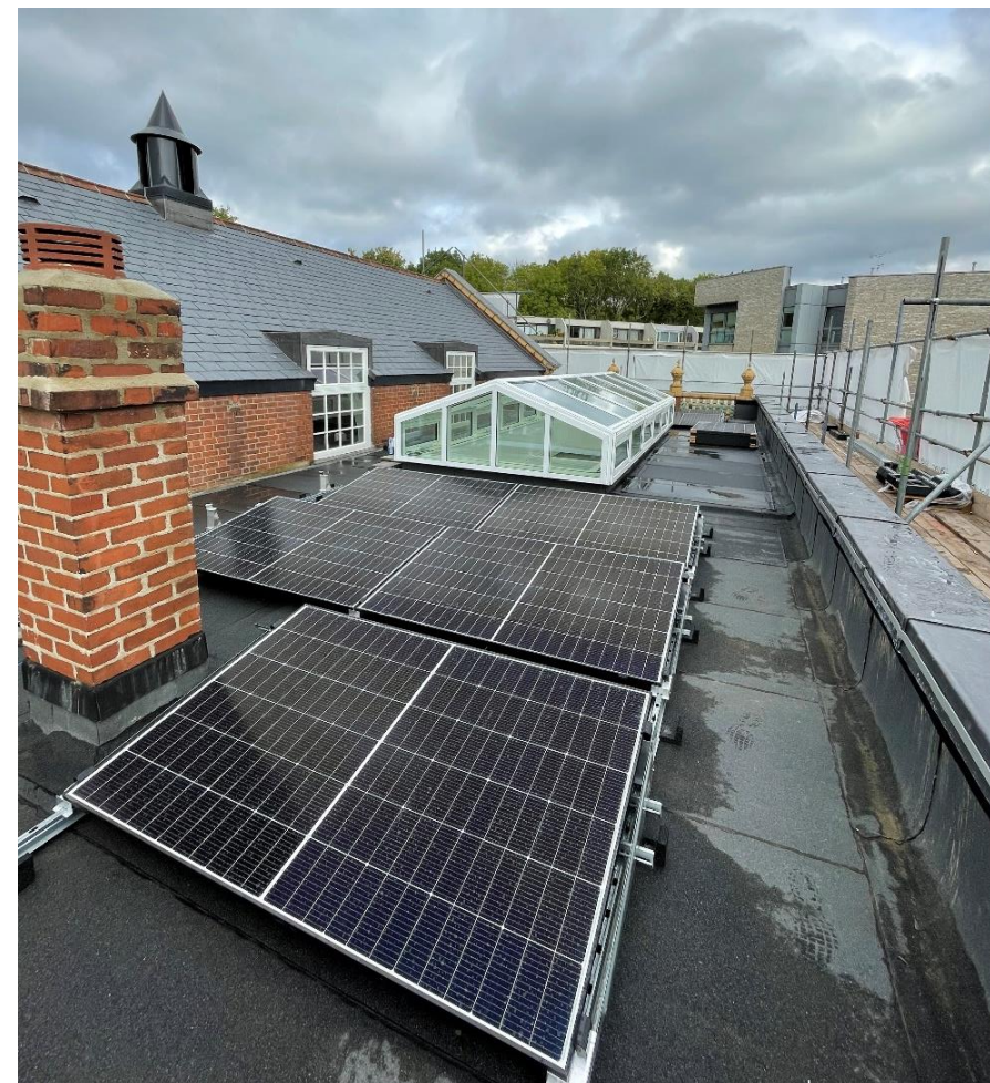
Figure 26: Solar panels installed on the roof of Highgate Library, as part of a whole-building retrofit project.
