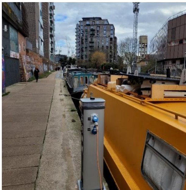
Figure 14: Electrical power supplies for ice cream vans (top) and canal boats (bottom).
