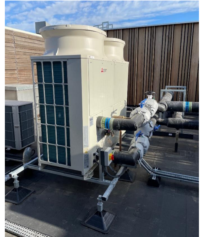
Figure 24: An air source heat pump installed at Talacre Community Sports Centre. This has replaced a gas boiler and will therefore reduce climate impacts whilst also helping to improve local air quality and protect community health and wellbeing.
